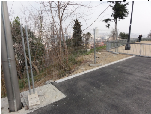
Illustration 45: Unsecured and unmarked construction site grid
