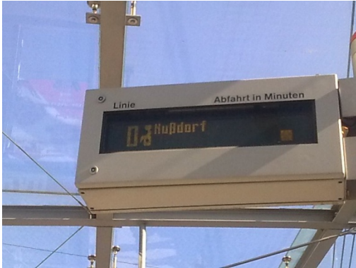
Illustration 10: Badly readable destination display in a station due to its low luminance
