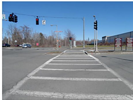
Countdown Signal at Signalized Intersection (2 sites)
